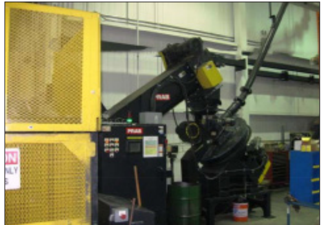
PRAB 24AD Wringer System (chips discharged to outdoor silo)
